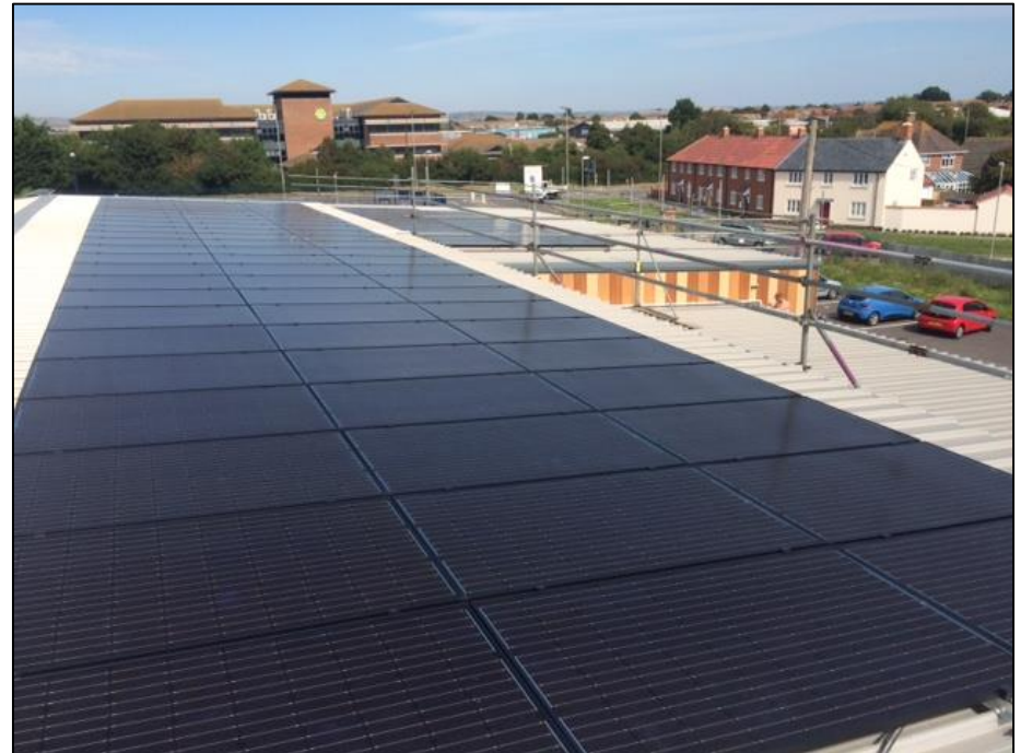
30kW of solar PV at Budmouth College
