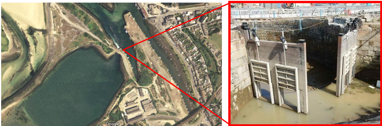
Figure 13 – Carnsew Pool sluice gates reinstated as part of the redevelopment at South Quay
