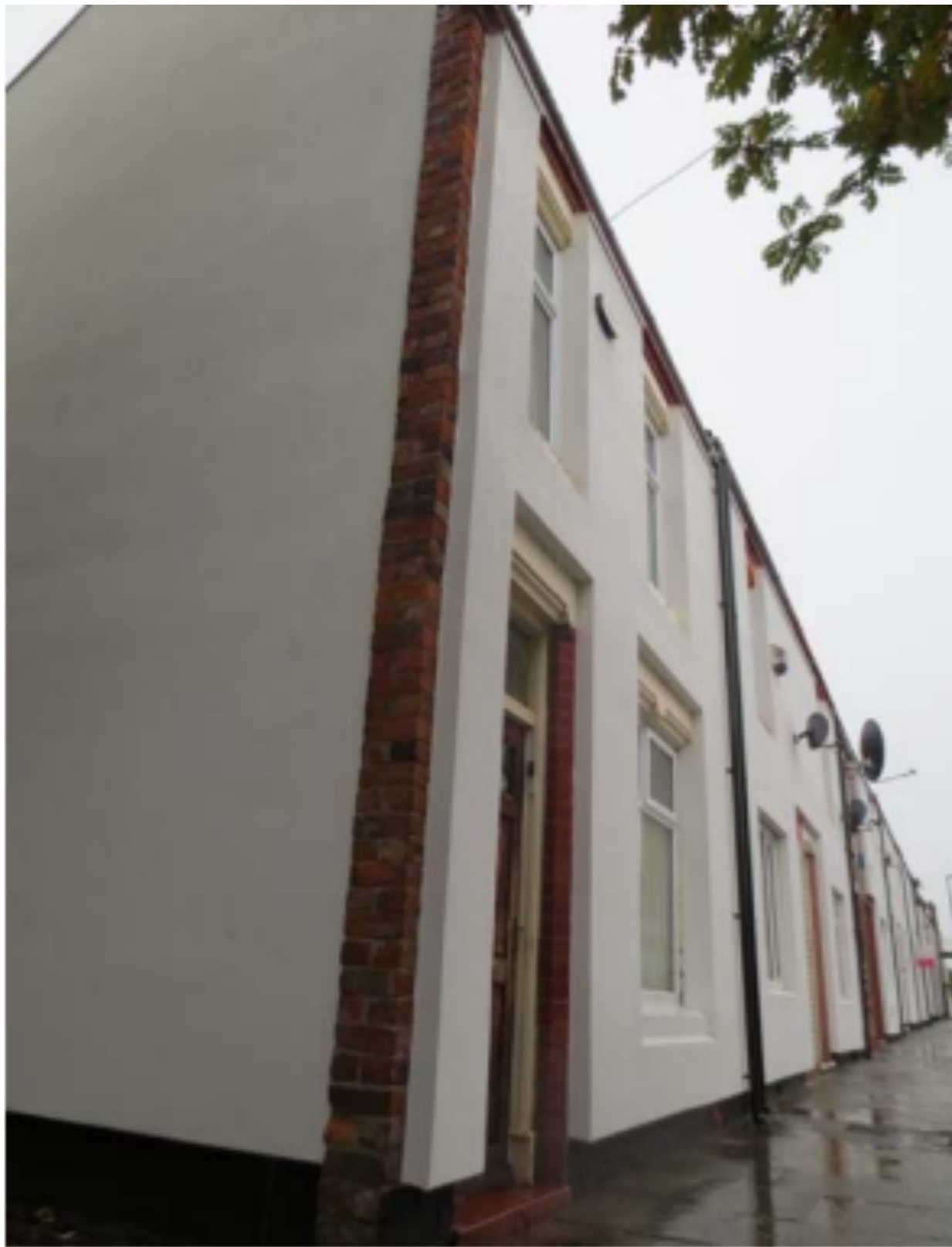
Figure 24 Note large areas of exposed building elements
