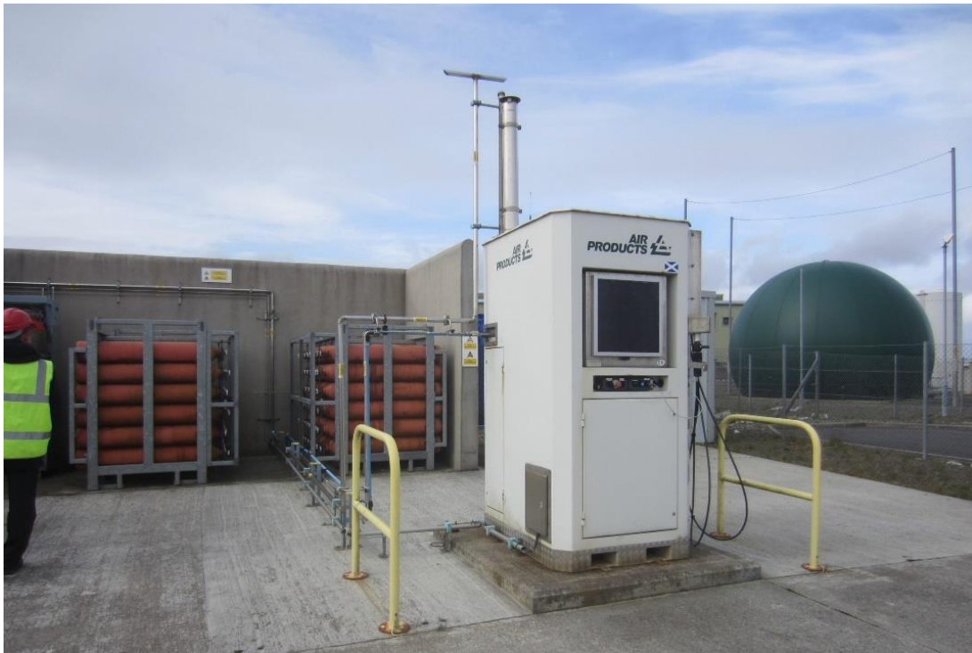
Figure 22 Outer Hebrides Local Energy Hub hydrogen store and refuel
